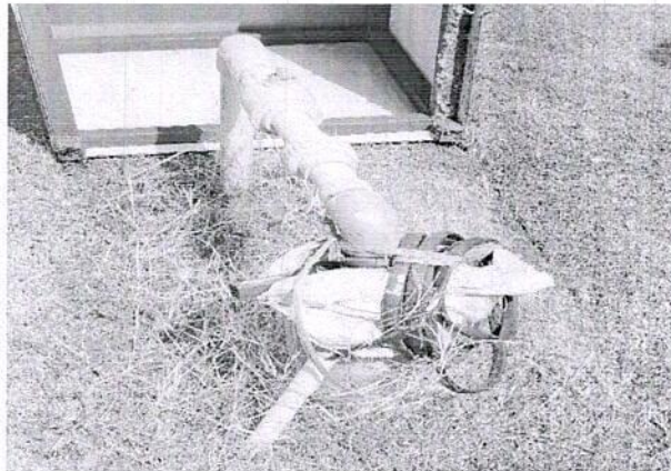
Pumping Set at IMS, Noida
