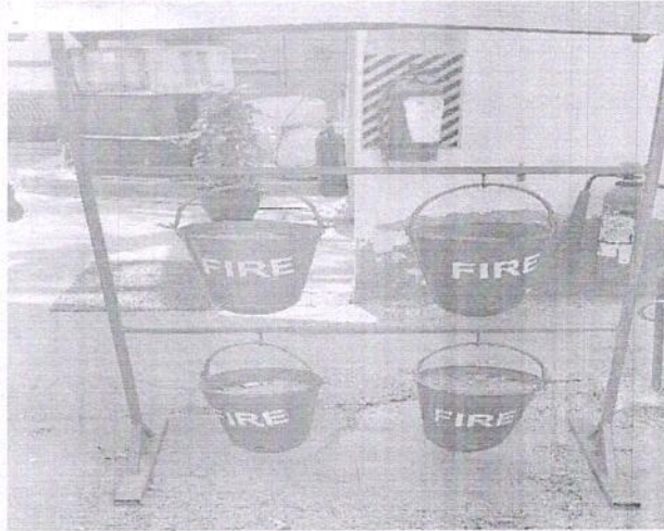
Provision for Fire Safety at IMS, Noida
